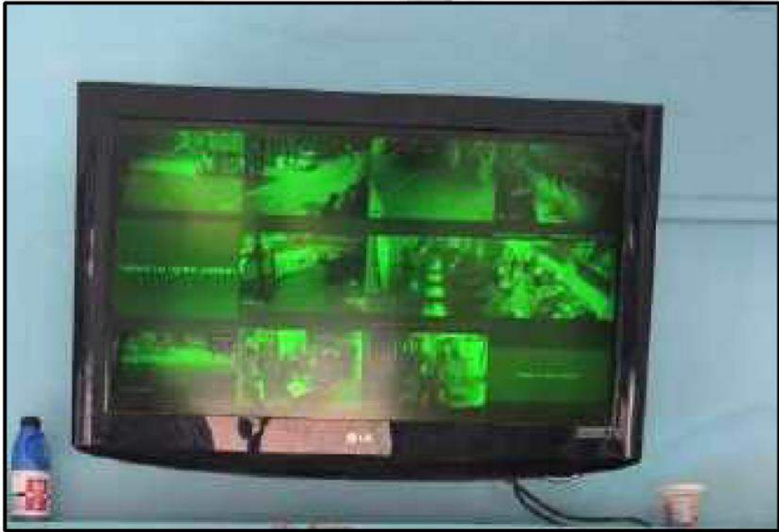
CCTV monitoring system
