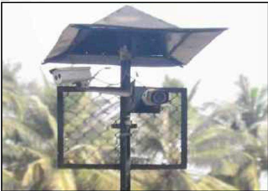
CCTV at the entrance
