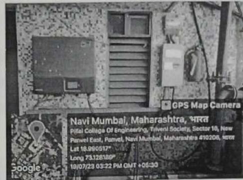
53.9 Kwp Solar Power Plant Invertors 25 Kwp Solar Power Plant Invertors
