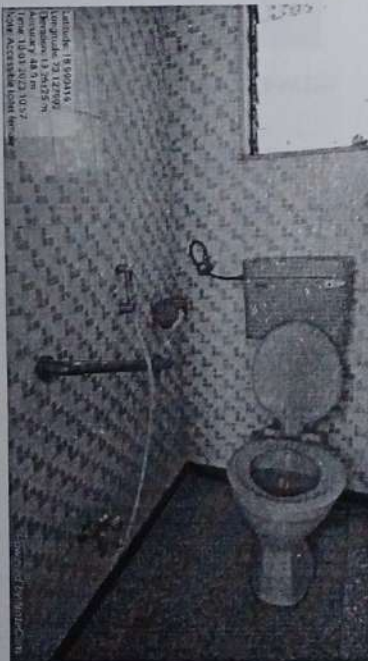
Internal view of toilet for Differently abled
