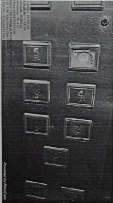
Signages in Braille on elevator
