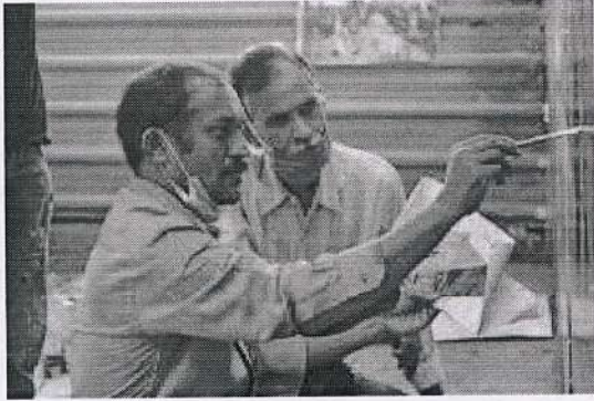
Students and staff painting the walls of New Panvel Railway Station as a part of the Beautification Drive
