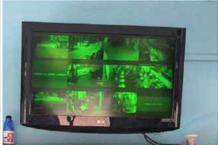
CCTV monitoring system
